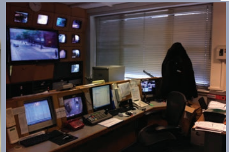
BEFORE: The cramped and oppressive control room prior to the refurbishment
