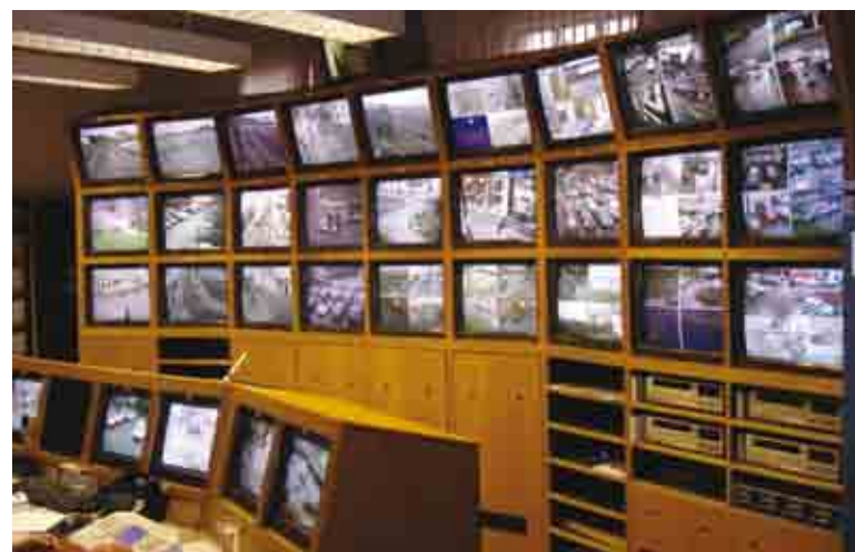
Before: poorly lit wooden control room
